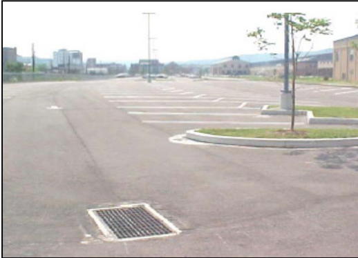
Grate Inlet in Parking Lot
